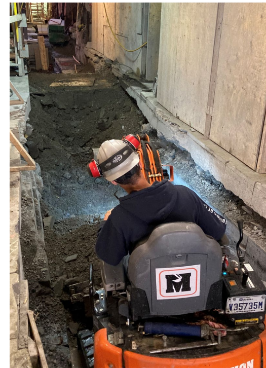
In the downtown powerhouse, construction is underway to electrify a natural gas boiler, which is anticipated to come online in 2023.
