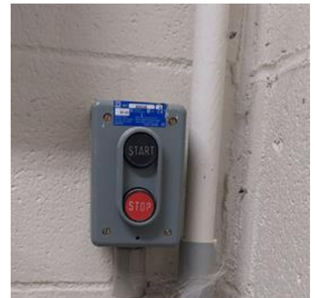
Figure 1. Manure pit control panel
