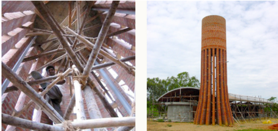
Figure 12 U.S. Pavilion Auroville, Tamil Nadu, India, 2002 A cistern and water tower to capture ,store and distribute the rainwater from the roof
