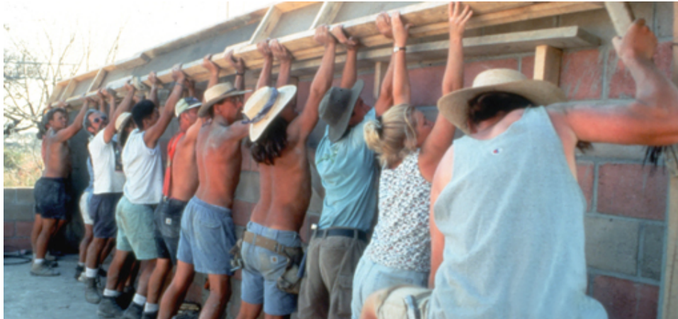
Figure 7 Escuela San Lucas Tejalpa, Morelos, Mexico 1995-1997 The community produced concrete block, pre-stressed pre-cast concrete beams, and infill blocks to build the structure.( the BaSiC Initiative)
