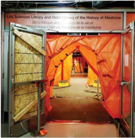
The entry to the library 3 weeks after the fire.
