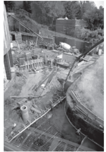
A New Neighbour. This photograph, taken earlier this year by Alan Forster, shows the groundwork for our new next door neighbour to the east of us, the Francesco Bellini Life Sciences Building and the new Cancer Research Pavilion
