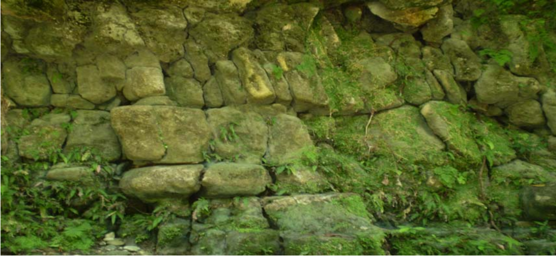
PICTURE 6 SHOWING LOOSE BLOCKS OF LIMESTONE ALONG THE JOINTS.
