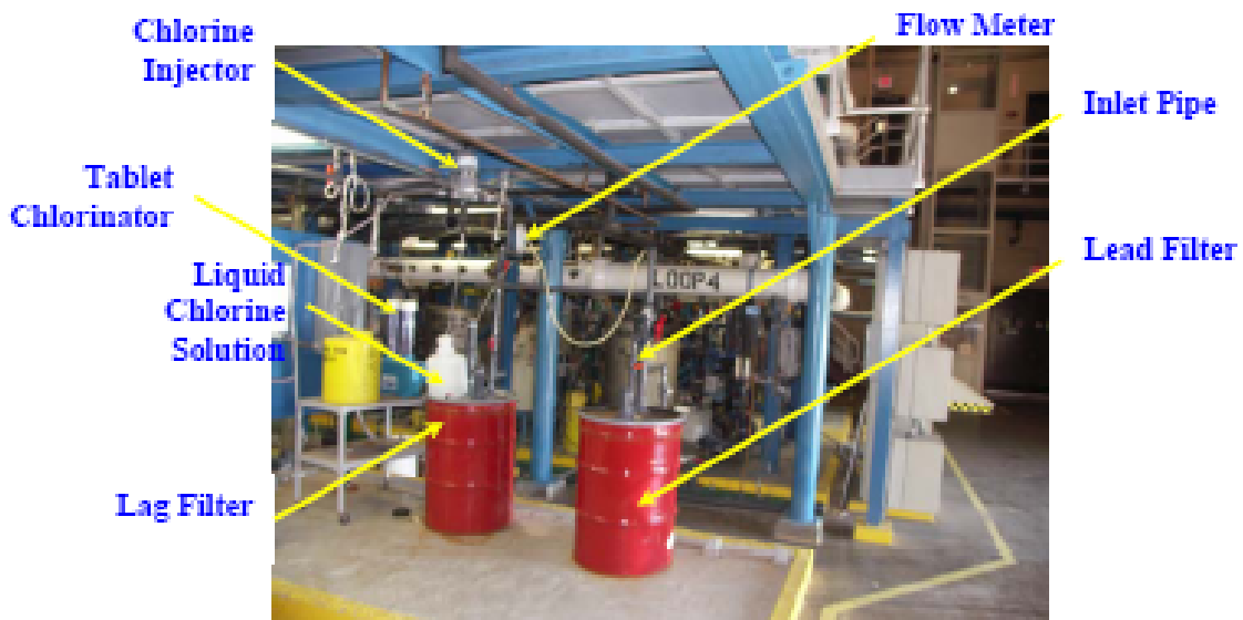
Figure 3. Drum filtration systems.
