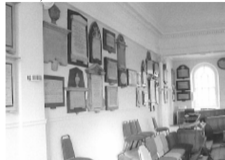
Missing plaques on west balcony wall., by kind permission of Chedburn Design-Architects
