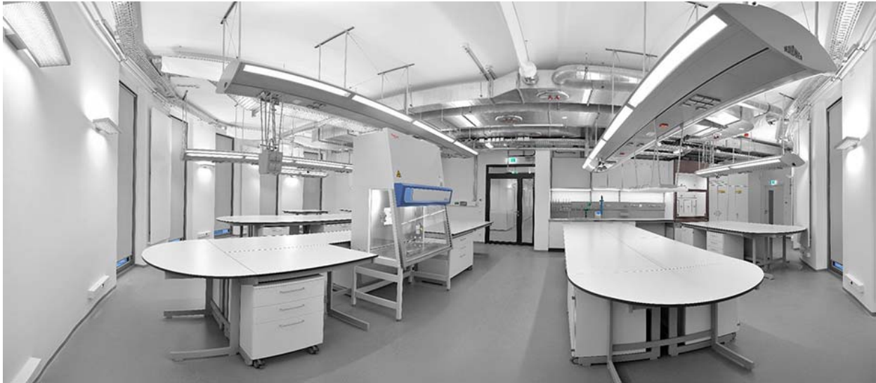
Flexible furniture with overhead service carriers, photo from Waldner Laboratory Systems
