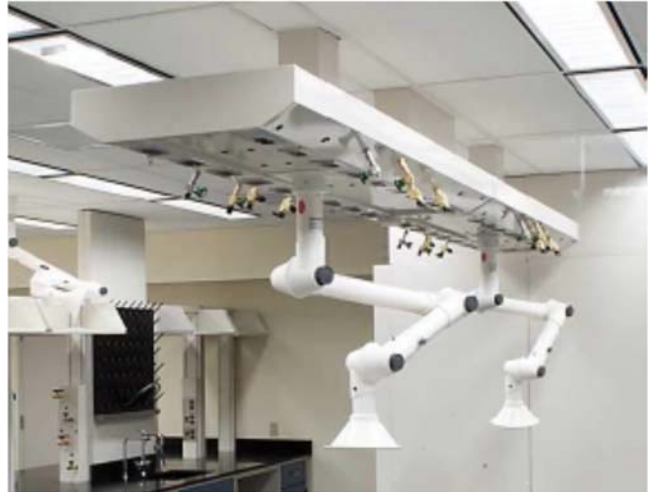
Overhead Utility Connections, photo from presentation by James Schreyer, From Afterthought to Forethought: Designing an Optimal Analytical lab
