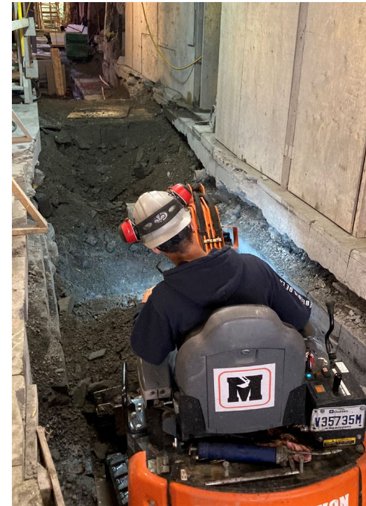
In the downtown powerhouse, construction is underway to electrify a natural gas boiler, which is anticipated to come online in 2023.
