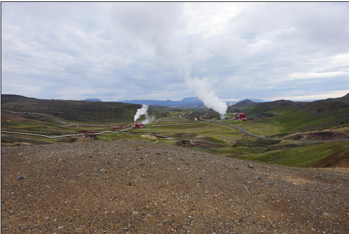
The geothermal powerplant inside Krafla caldera
